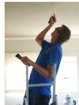
Auke Bergsma in 2014, helping with the finishing of building the Youth Centre during his visit.
